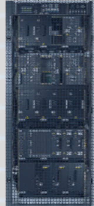
Multi-standard Base Station GSM/GPRS/EDGE/UMTS (ALU)
