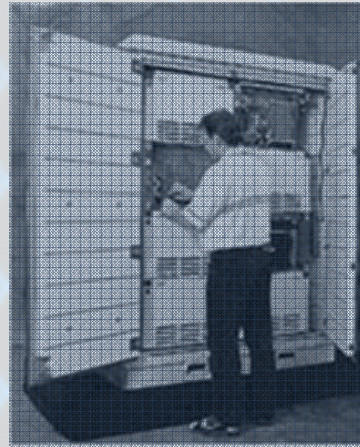
Dual band IS-136 RBS 884 Base Station (Ericsson)
